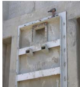
STUCK CEMENT (OVER 12 FEET)
